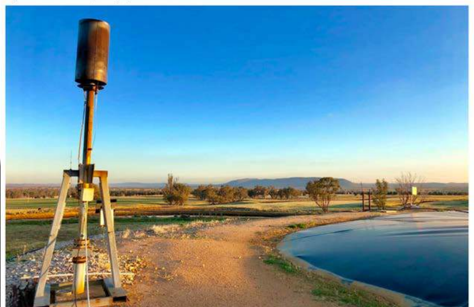
Figure 31 – Indicative photograph - methane flare
